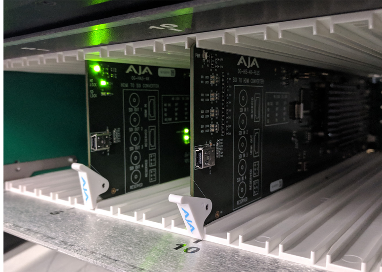
Figure 7. Card on Right Not Fully Inserted
